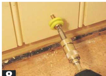
8 Remove markers, then drill and screw buttons to panelling. Click skirting in place and adjust if necessary
